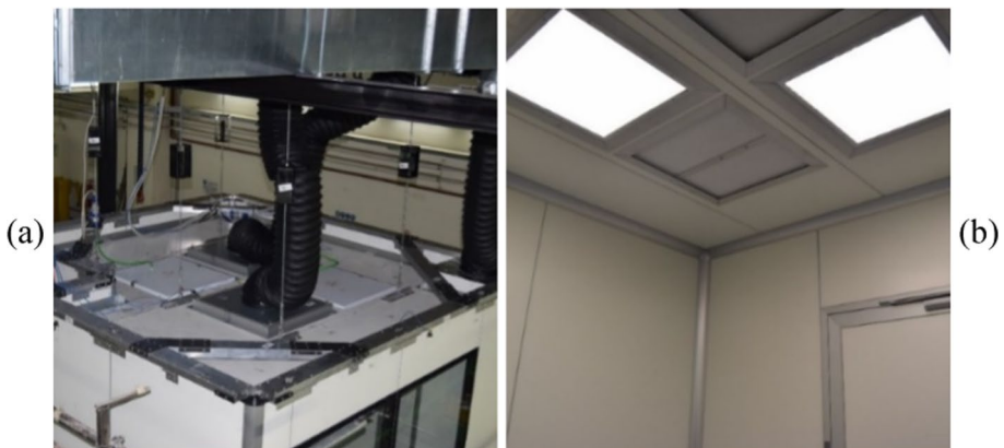
Fig. 4 View of the assembled ceiling system: a from the top and b from the inside the cleanroom
