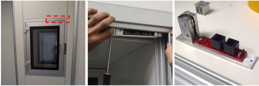
Fig. 10 Damage of the electromagnetic lock of the inside door of pass-box, ID 110 test
